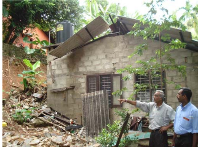
A house destroyed by a cyclone
